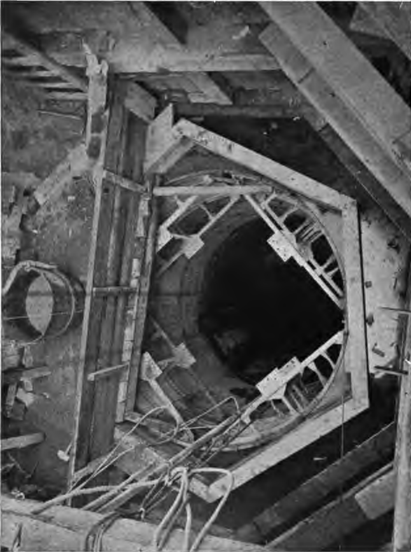
PLATE 214.—View Looking Down Shaft, Showing Timbering for Chamber to Rock and Concrete Lining in Rock Shaft Below. Steel shaft form—Blaw—in place at top.
